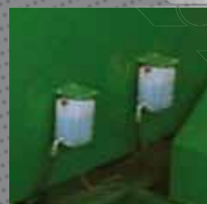
Tanks for mantening oil at gear boxes.
