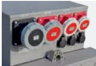
Switch box for variants Feed into the building IT / TN
